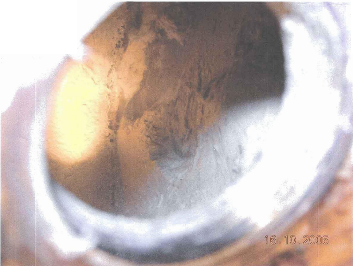
photo 5: the internal status of the steam drum before “active water generator” fixed
